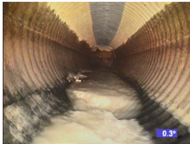
Photo 31 – View of a corrugated double wall HDPE pipe with minimal slope (0.3°), which was so slick that access with inspection equipment was severely limited.
