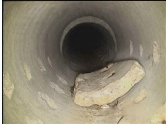
Photo 75 – View of a piece of a broken crown which permanently obstructed access.
