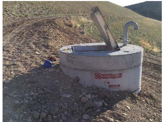
Photo 37 – An inspection well constructed next to an upslope access road, and low enough to allow easy access for inspection and maintenance equipment.
