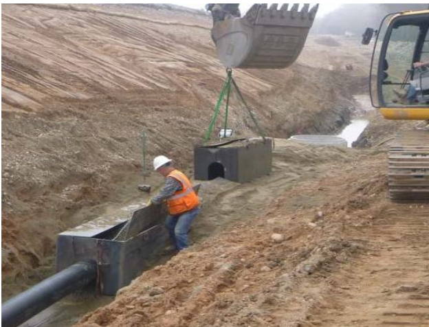
Photo 66 – View of contractor using slipform shoring panels to construct a two-stage filter. Notice the filter will have a trapezoidal sand filter and a rectangular drainage material cross section.
