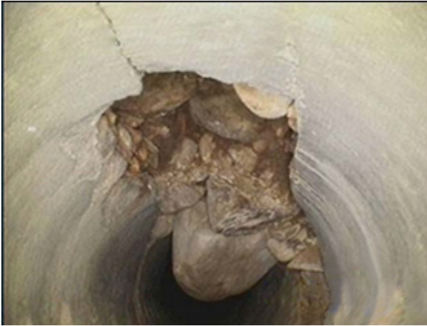
Photo 74 – Damaged crown of an outfall pipe that prevented inspection access of the toe drain.
