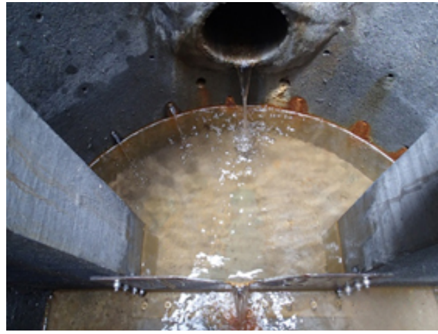
Photo 47 – View of perforations on upstream side of inspection well to capture as much seepage as possible.
