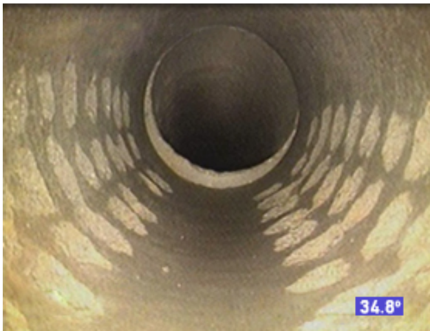
Photo 30 – View of inspection equipment accessing a steep (34°) abutment drain. Access was ultimately limited by a significant change in slope, and subsequent offset, at the top of the incline.
