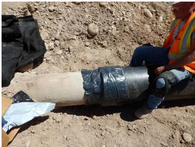
Photo 24 – A broken portion of 10-inch-diameter concrete toe drain pipe being replaced with concentrically-placed 12-inch-diameter HDPE.
