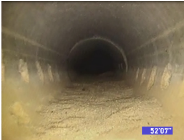
Photo 72 – Slope of conduit continues to decrease, while depth of sediment increases.
