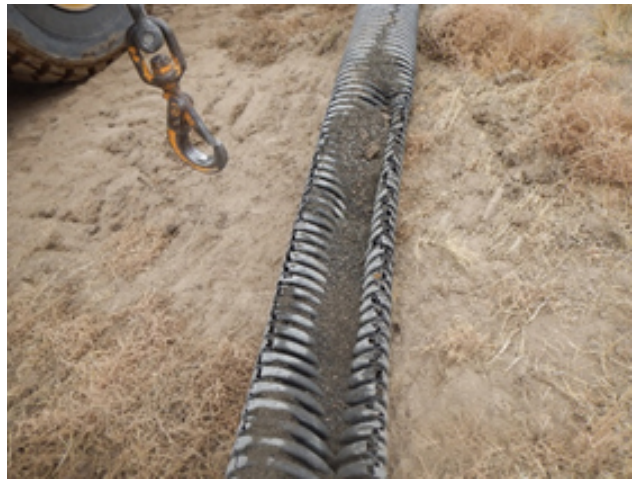
Photo 19 – View of a buckled corrugated HDPE drain pipe, likely caused from vehicular traffic traversing the drains.
