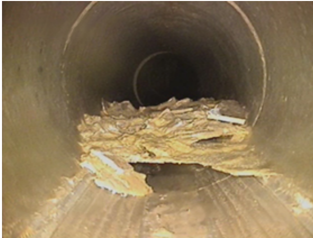
Photo 10 – Mineral encrustation created a permanent obstruction preventing inspection access.
