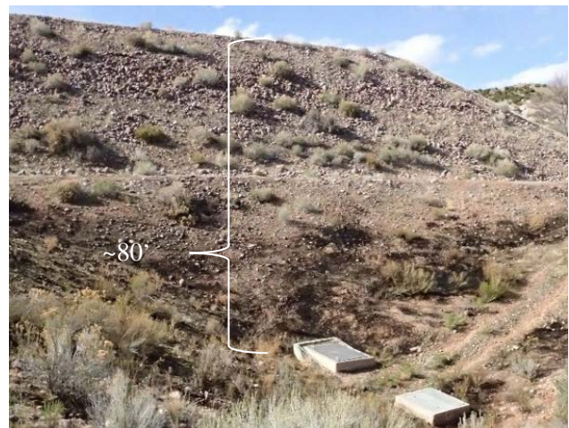
Photo 39 – View of a seismic berm constructed over the existing toe drains, placing over 80’ of material above the drains.
