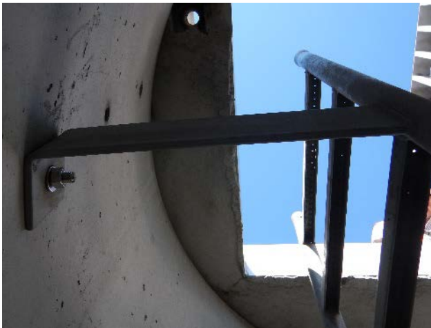
Photo 44 – Ladder rungs extending 16” from the inside wall (rather than 7”), ensuring that the extendable safety rail clears the hatch.
