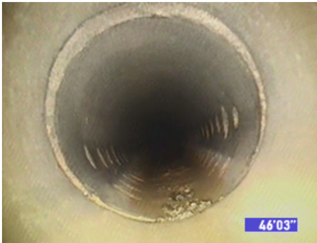
Photo 70 – View of a joint opening which allowed seepage to dissipate. Notice signs of water level in the upstream conduit.
