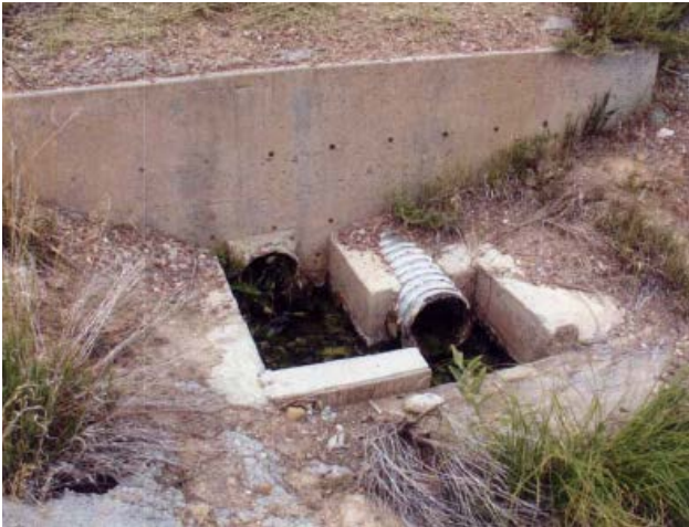
Photo 50 – View of an unprotected settling basin at the outfall of a toe drain system.
