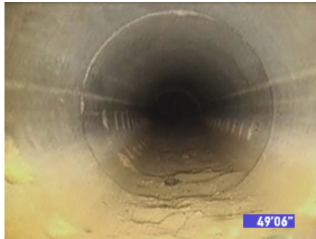
Photo 71 – Sediment gradually accumulates as the slope of the conduit decreases.
