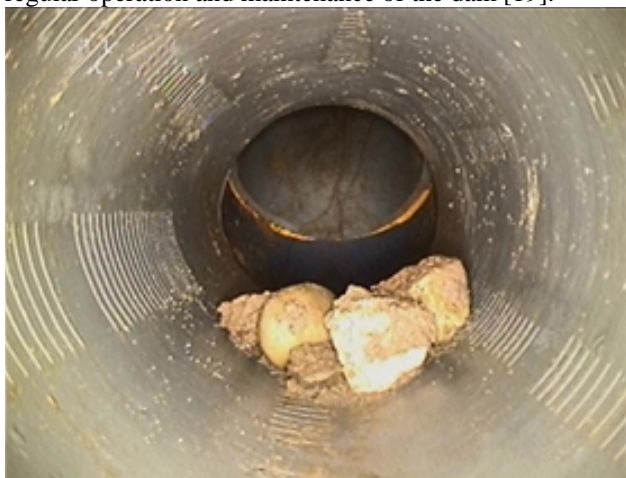
Photo 8 – View of gravel at the base of a cleanout, likely introduced during construction, creating a permanent obstruction for inspection equipment.
