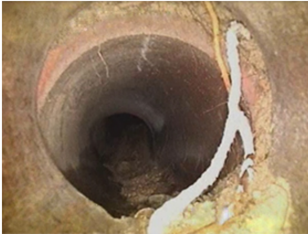
Photo 28 – Offset in a clay tile pipe which prevented further inspection of the toe drain.
