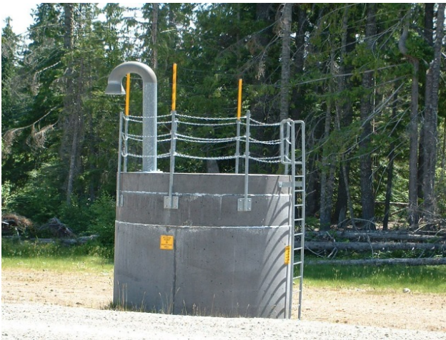
Photo 36 – An inspection well constructed to this height would create substantial friction on both the inspection and maintenance equipment.
