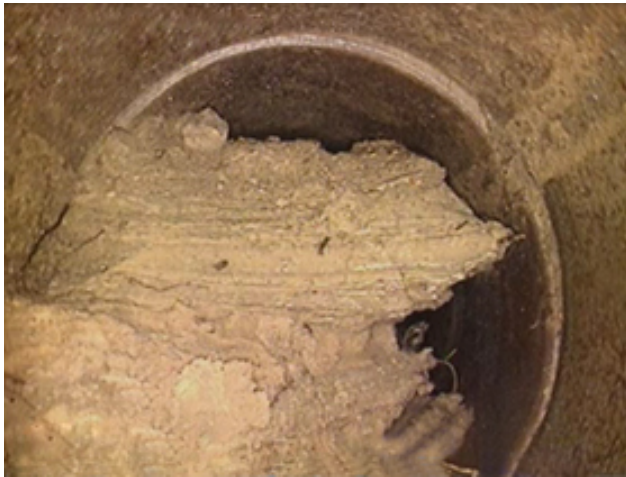
Photo 22 – View of a pipe that was completely full of sediment. Notice the stratification of sediment indicating that material movement and deposition has been occurring slowly over time.
