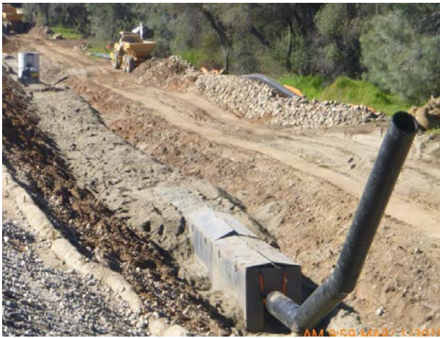
Photo 52 – View of two 22.5° bends coupled to provide a cleanout at the upstream terminus.
