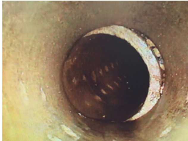
Photo 29 – Offset in a concrete pipe which prevented further inspection of the toe drain.
