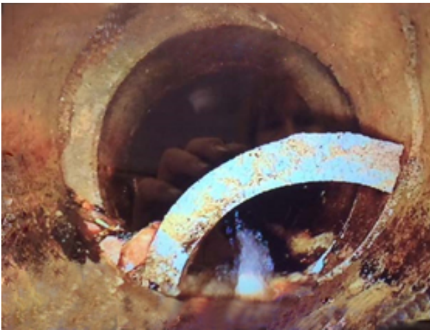
Photo 64 – View of a broken crown of a drain pipe that was lodged during modification of the toe drain.
