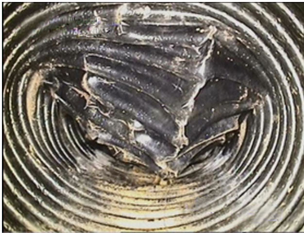
Photo 18 – View of a buckled corrugated HDPE drain pipe.
