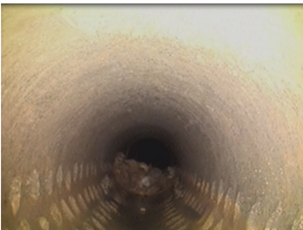
Photo 3 – View of a gravel pile obstructing access in a toe drain.
