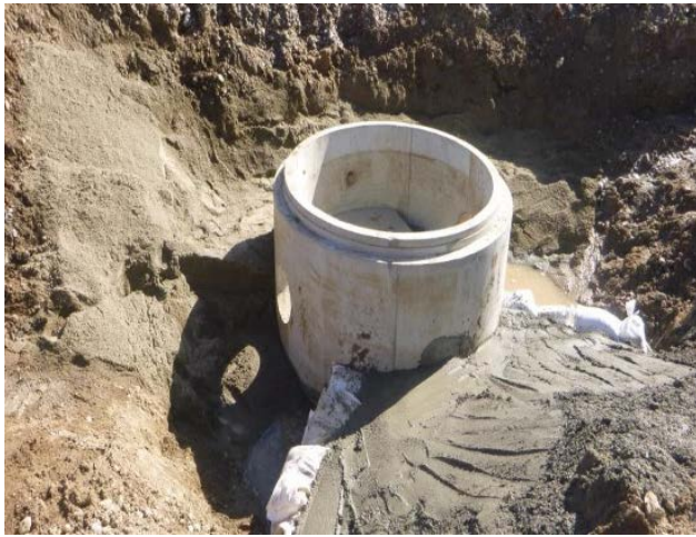
Photo 46 – View of a downstream CLSM berm used to force seepage into inspection well and drains.
