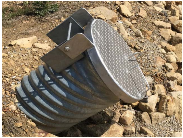
Photo 53 – View of a typical cleanout and lid installed at the upstream terminus of a toe drain system.
