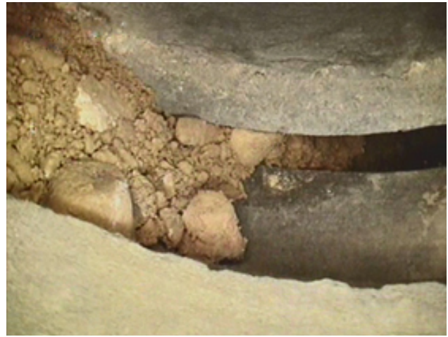
Photo 69 – View of material accumulated on the invert of the pipe due to another large joint opening.
