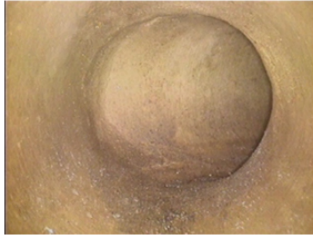
Photo 41 – View of a 90° elbow in 24-inch pipe. Inspection equipment navigated this bend well enough, but the jetter could not due to its inability to steer.
