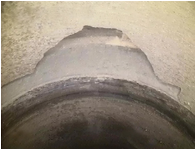
Photo 16 – Broken area near the crown of a bell-and-spigot connection between sections of concrete pipe, caused during construction.
