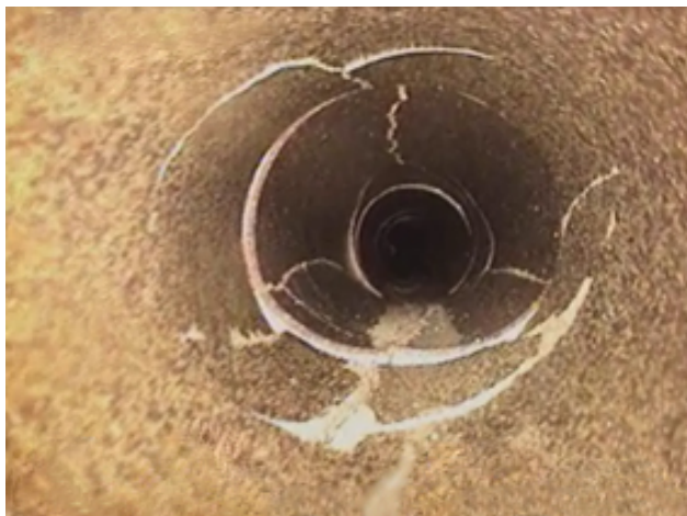
Photo 14 – Cracked clay-tile pipe.
