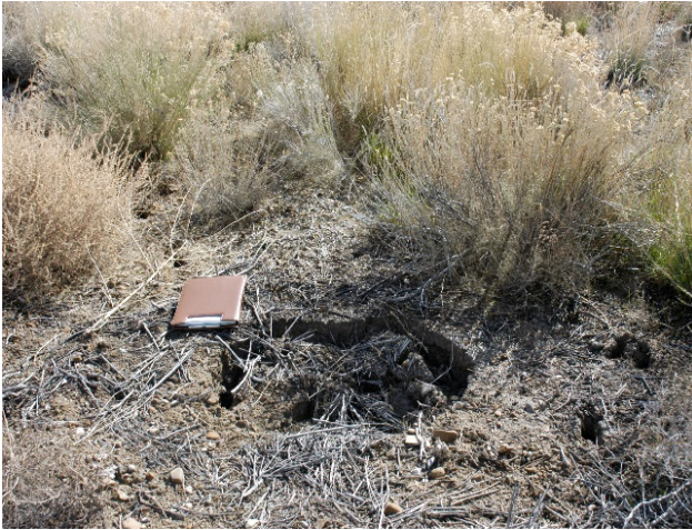
Photo 40 – View of a sinkhole which formed above a toe drain outfall pipe with large perforations and no filter.
