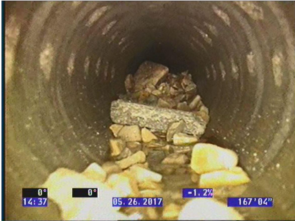
Figure 5: Large Blockage around 170 feet
