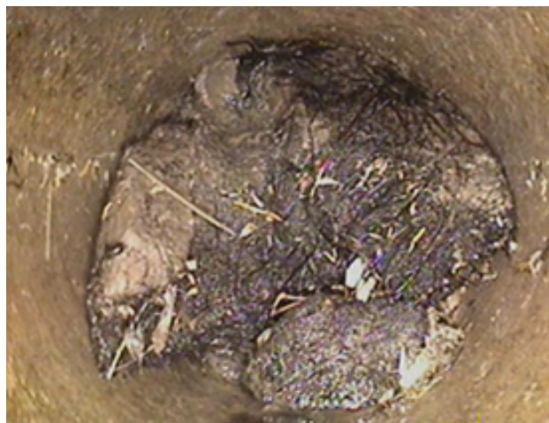
Photo 9 – View of a root-ball completely plugging a drain.
