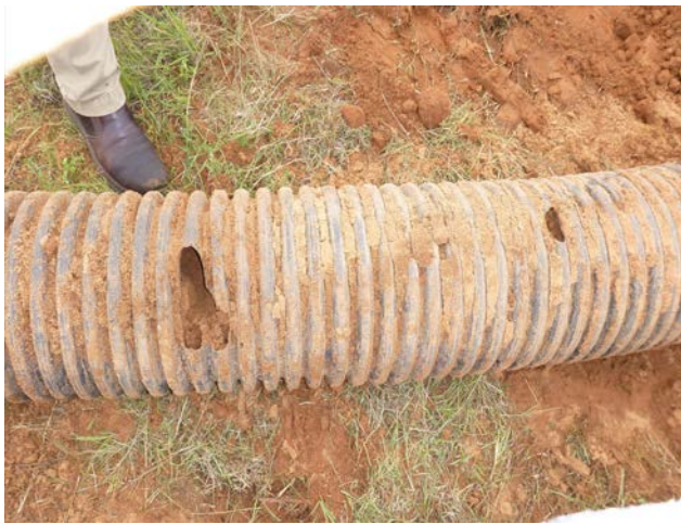
Photo 20 – View of holes caused by rodents burrowing through a single-walled HDPE pipe.
