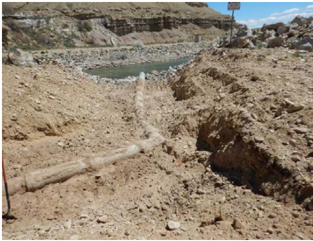
Photo 34 – A sharp bend in a toe drain outfall pipe which prevented inspection and cleaning equipment access.
