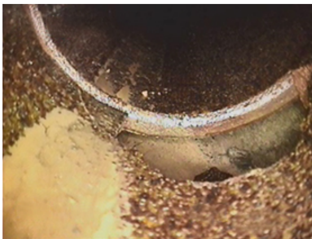
Photo 6 – View of a gap near the invert of a drain outfall, exposing the surrounding material.
