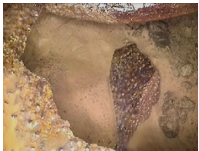
Photo 7 – A jetter quickly eroded out material in this area and developed a much larger hole.
