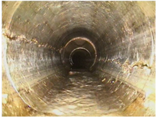
Photo 17 – View of longitudinal cracking in a concrete pipe, caused by overburden pressure.
