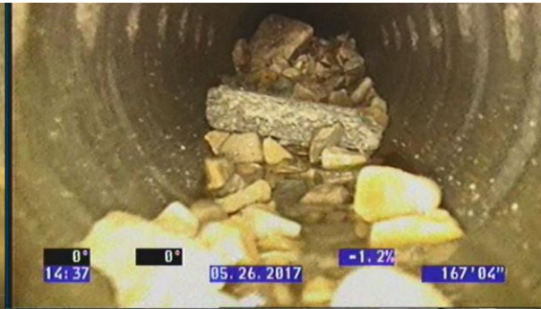
Figure 2: Blocked portion of pipe at 170'
