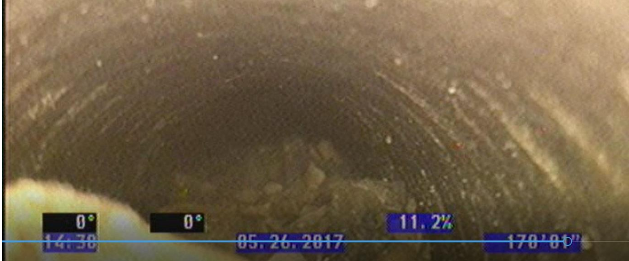
Figure 7: Zoomed in image showing further blockage behind large blockage at 170 feet
