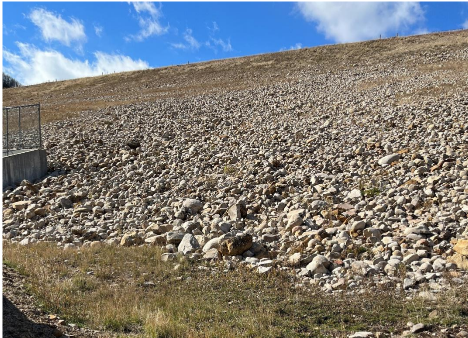
Figure 4: Little plant growth on the left face of the dam
