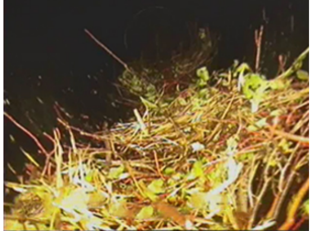
Photo 61 – View of a rodent nest blocking inspection access to the rest of the drain.
