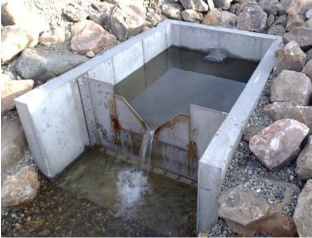
Photo 48 – View of water backed up into a toe drain system because of the measurement weir configuration.
