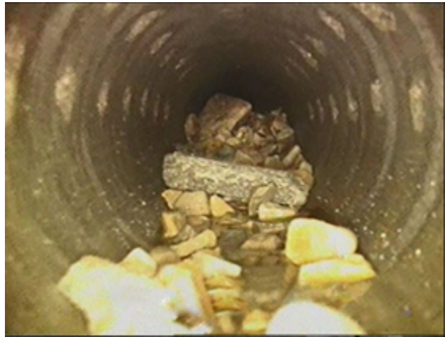
Photo 65 – Portion of crushed pipe and gravel sized material, blocking inspection.
