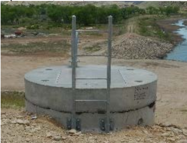
Photo 42 – Permanent ladder extension mounted on the exterior of an inspection well.
