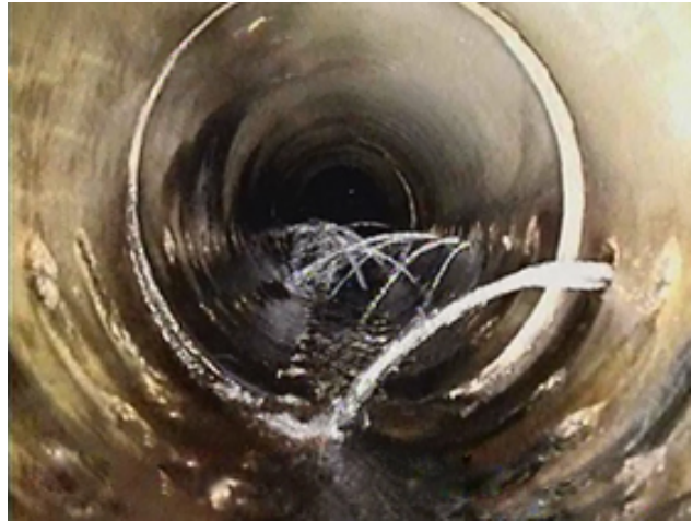
Photo 11 – Pressurized water entering through some of the perforations, while others are plugged up by sediment or mineral encrustation.
