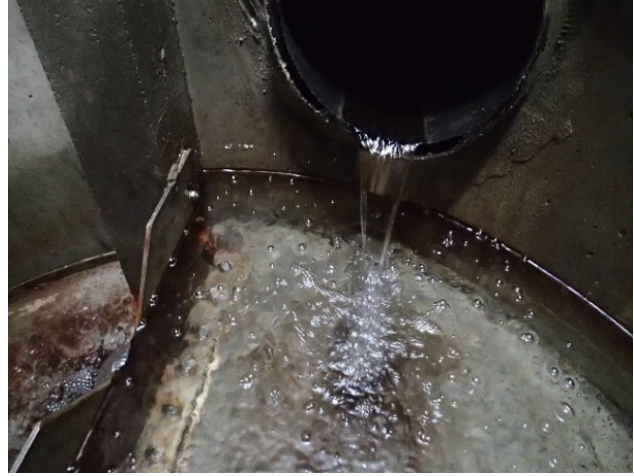
Photo 49 – View of a free-flowing toe drain outfall with sufficient distance between the pipe and weir inverts.
