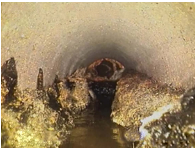
Photo 12 – View of biofouling along an abutment drain prior to cleaning.
