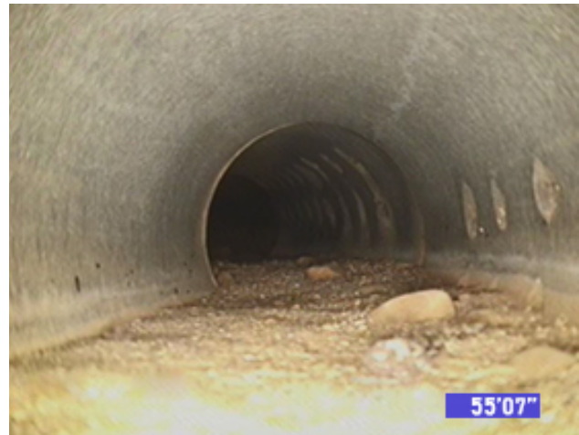
Photo 73 – View of the sediment deposits and high water level.
