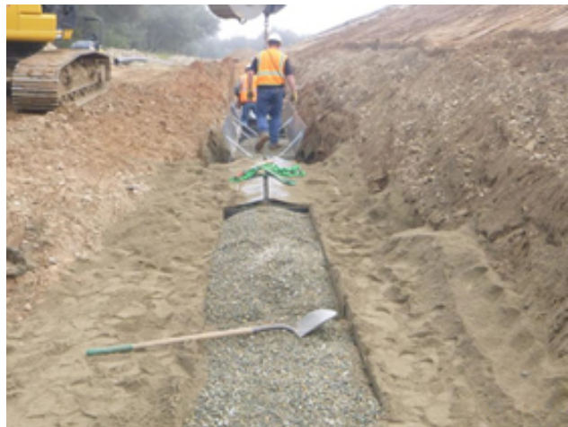
Photo 67 – View of a trapezoidal two stage filter with a rectangular drainage material zone using slipform shoring panels (similar to design in Figure 4).
