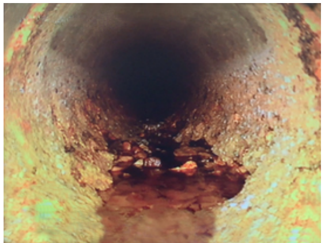
Photo 13 – View of a deteriorated invert of pipe, similar in location as that shown in Photo 12, after biofouling was removed.
