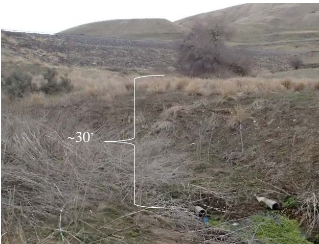
Photo 38 – These toe drains were buried almost thirty feet below the base of the toe, and would require significant excavation into the embankment to replace the drains.
