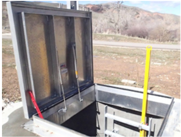
Photo 43 – View of a manhole lid with hydraulic supports and an extendable grab bar.
