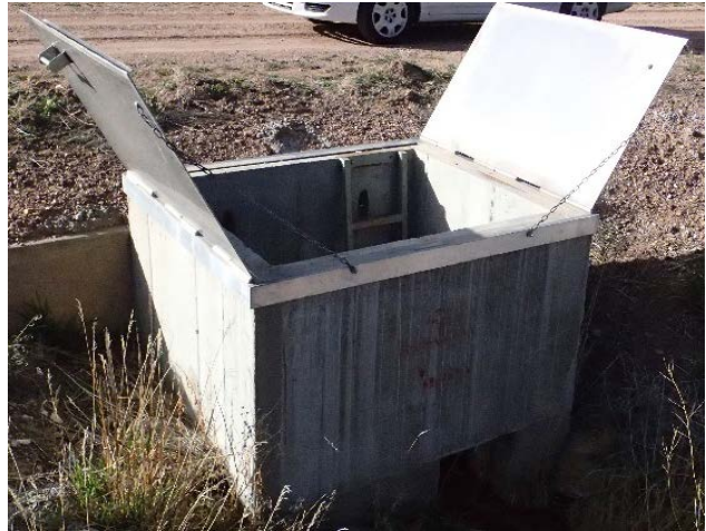
Photo 51 – A vault was constructed around the settling basin shown in Photo 50 to prevent foreign material from entering.
