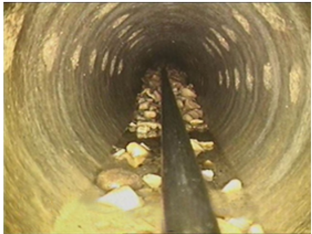
Photo 23 – View of a gravel pile in a 10-inch pipe that was large enough to completely lodge a jetter head, requiring mechanical extraction.
