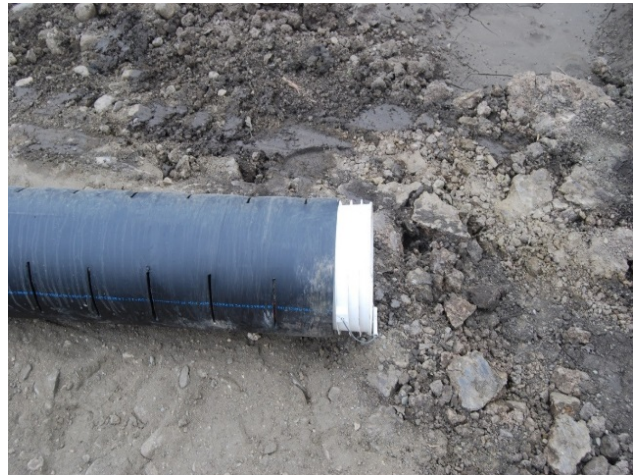
Photo 55 – View of a temporary drain end cap using a generic five-gallon bucket.
