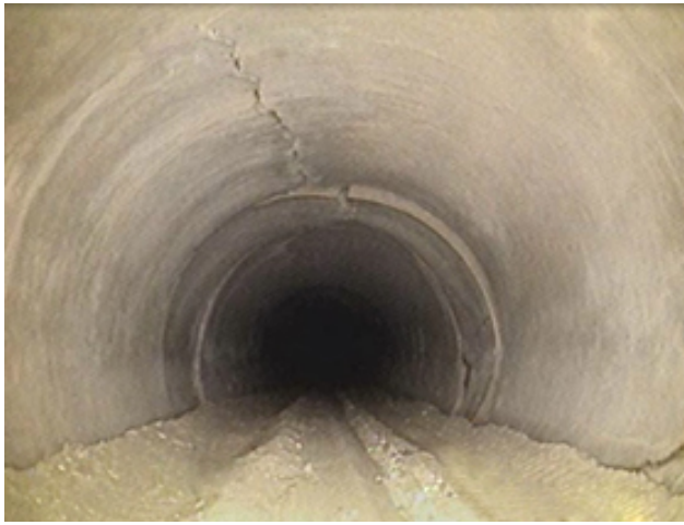
Photo 56 – View of sand deposits in the toe drain outfall.
