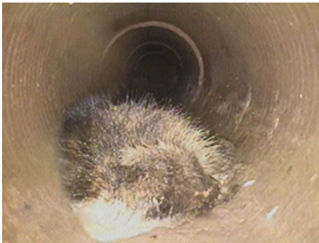
Photo 62 – View of a deceased rodent blocking inspection access to the drain.
