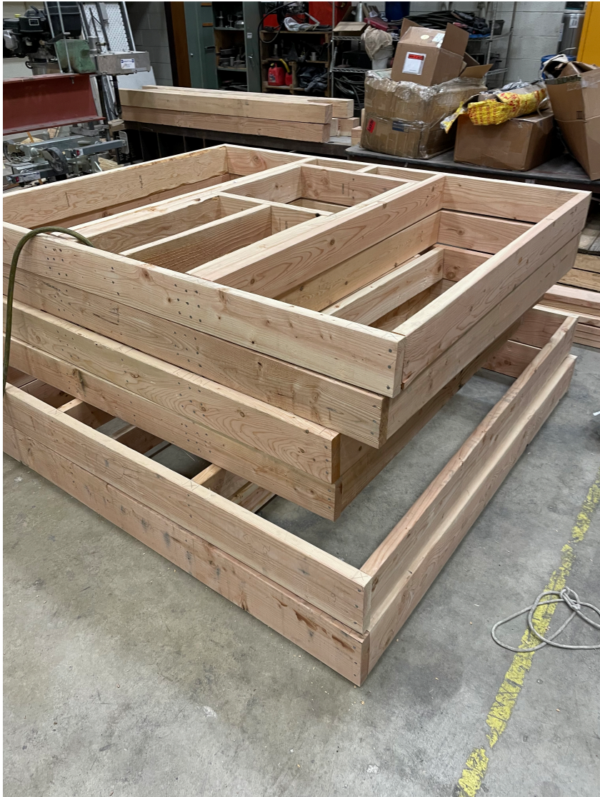
Figure 7 An image of several floors and walls, all framed and ready for sheathing!
