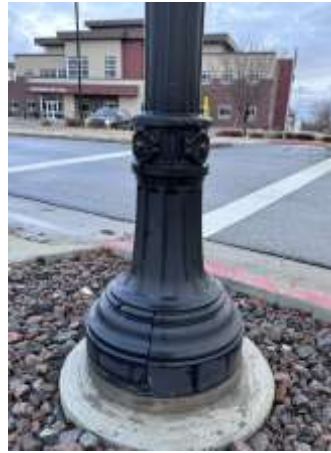
Figure 5: Common Light Pole 2
